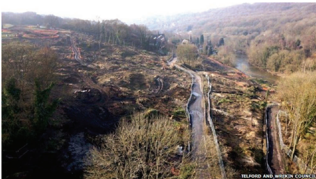
Figure 15: Work to address land instability between Jackfield Tile Museum and Boat Inn
